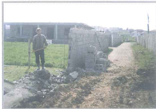
Consensual removal of the private fences to make room for public spaces and roads
