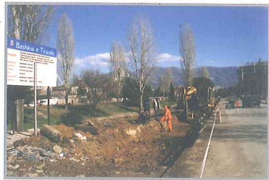
View of the demolition of illegal kiosks and constructions in the sides of Lana
