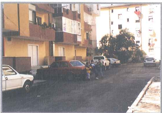
Refurbishment of public spaces in the so called Block "1 May", where community contribution was 20 % of total project cost. (from up to down situation before, during and after the project)
