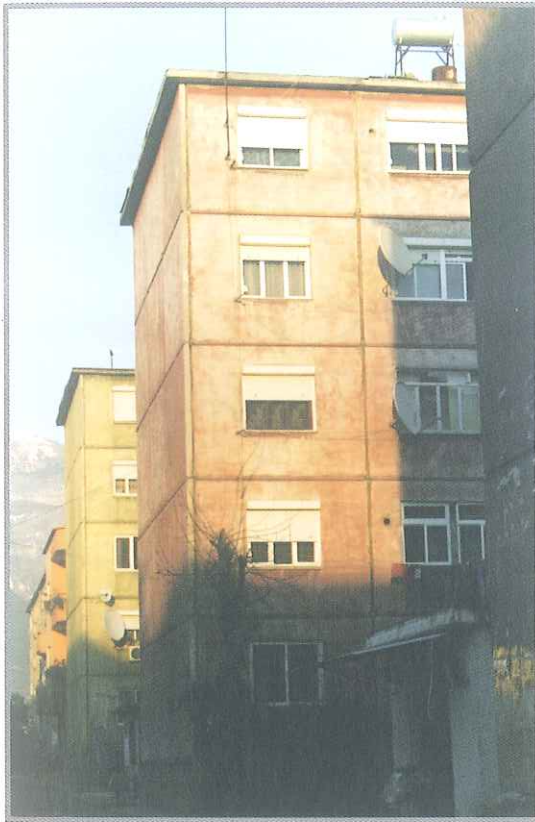
A line of flat building units based on pre-fabricated armed concrete elements
