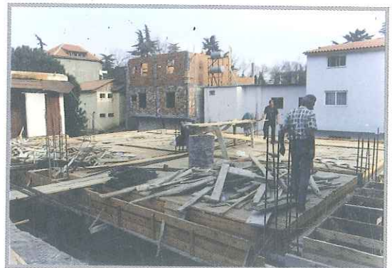
A process of illegal construction in the side and over Lana river
