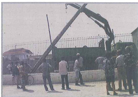
Installation of energy infrastructure in "Breglumas" where 95% of the community has paid the financial contribution.
