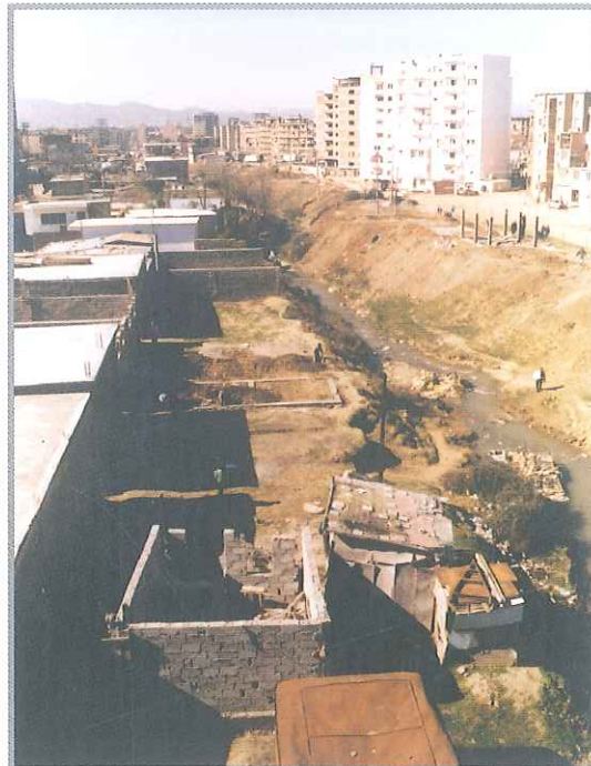
Degradation of the bed and sides of Lana river from illegal construction
