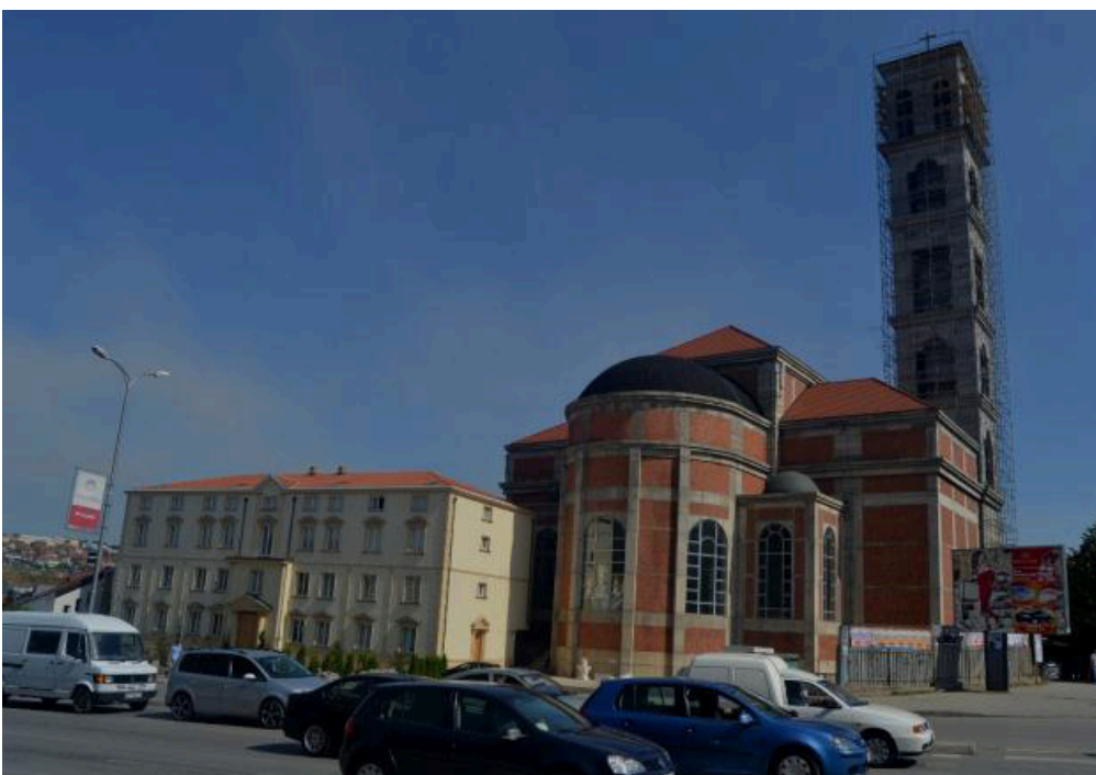
Figure 2: Works completed up to now on the construction of the Mother Theresa Cathedral in Pristina, 2012
