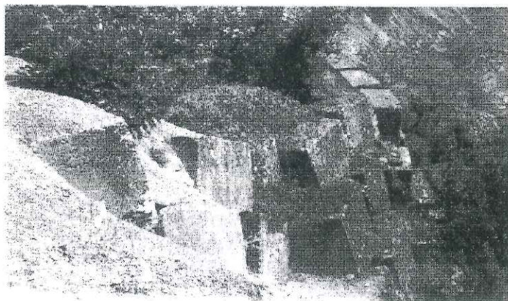
Fig. 8 Bogova landslide. It's looking to east, and shows, a destroyed retaining wall (deformed) by mass movement
