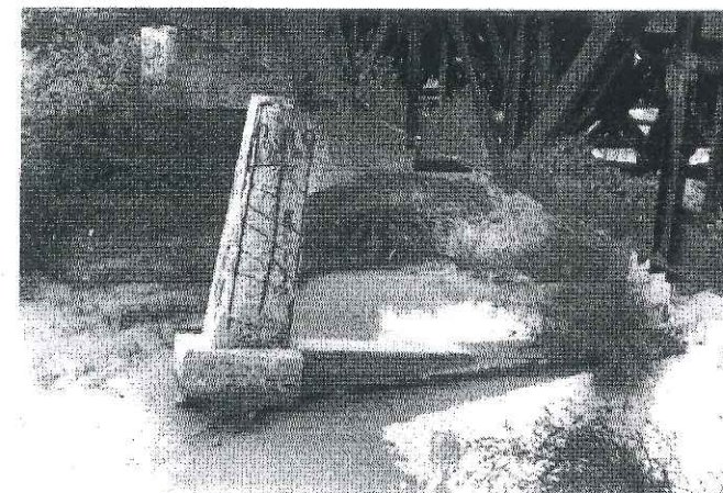
Fig.4 Mifoli bridge. It's looking to north and shows the sinking of its pier
