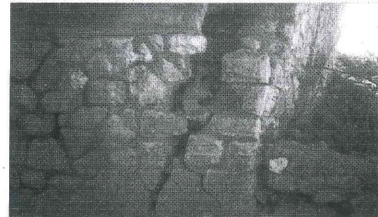
Fig.7. Kallmeti bridge. It shows cracks of pillars from erosion phenomenon
