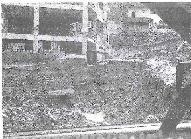
Pile wall failure (metallic proper failure)
