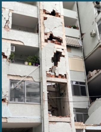
Fig.5 Significant damage to the building with high flexibility
