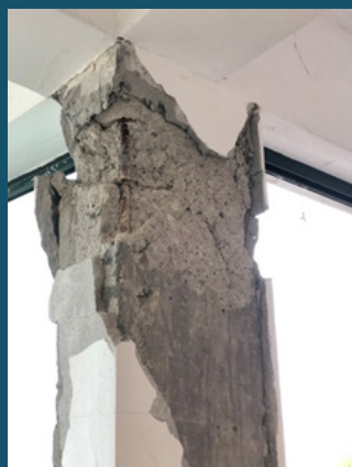
Fig.4 – Structural damages, plastic hinges on columns
