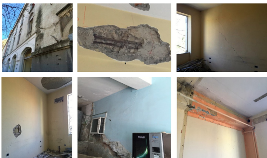
Fig 2. Damages of MZHU building
