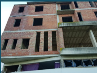
Fig.3 Structural damages, plastic hinges on columns.
