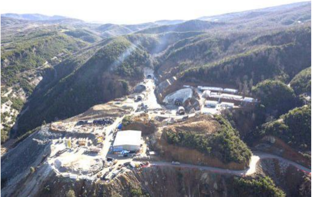
Fig1 / the New Highway Tirana - Elbasan under construction from KLM 2+850 (distance counting starting from Tirana) up to the Entrance of the Krabe Tunnel KLM 15+650 / source AKTOR
