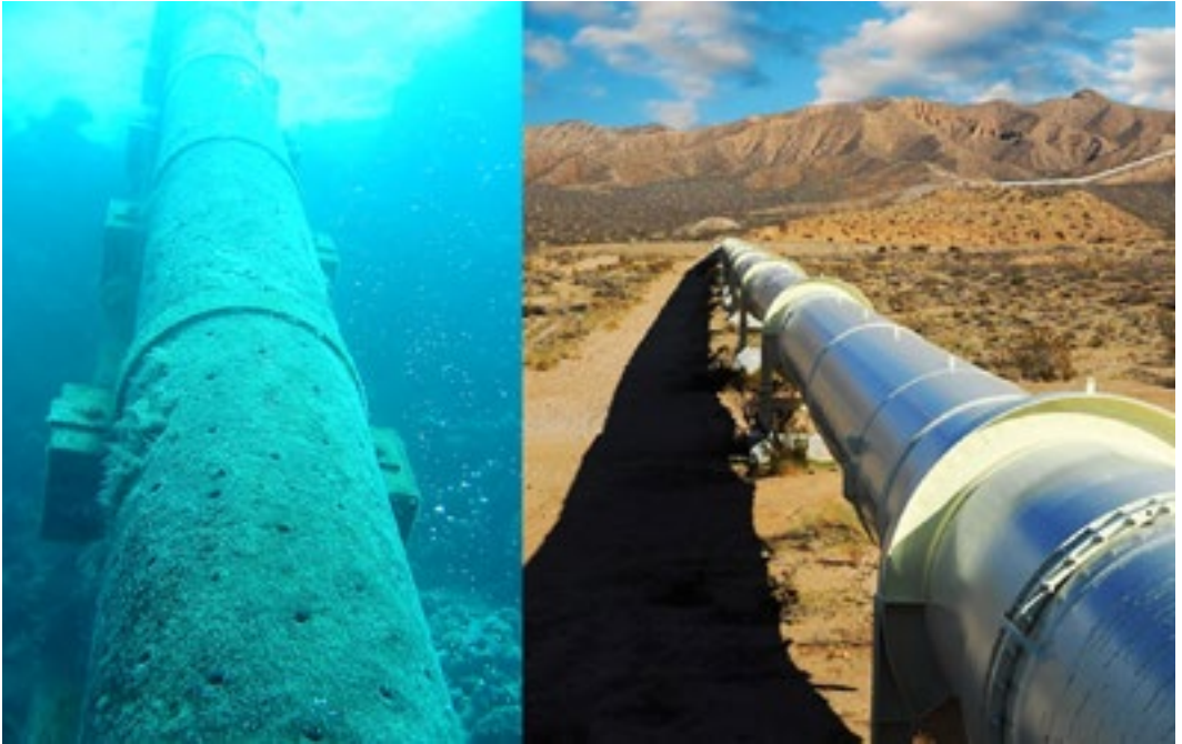
Fig3 / the Trans-Adriatic Pipeline (TAP), under construction, will connect with the Trans Anatolian Pipeline (TANAP) at the Turkish-Greek border at Kipoi, cross Greece and Albania and the Adriatic Sea, before coming ashore in Southern Italy / source internet
