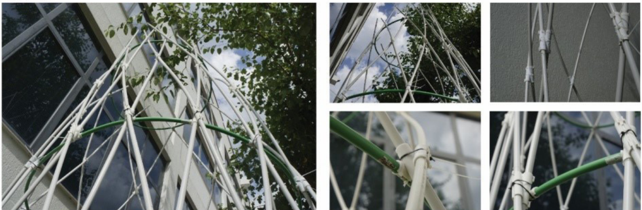
Figure 8 Assembly process of the PVC pipe structure and details photos: author and Sara Codarin
