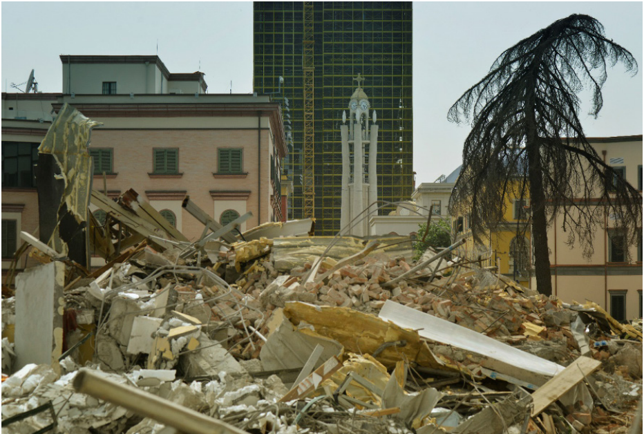
Figure 8: The ruins of the National Theatre, a few moments after the collapse, 17 May 2020. Courtesy of the author Artan Rama
