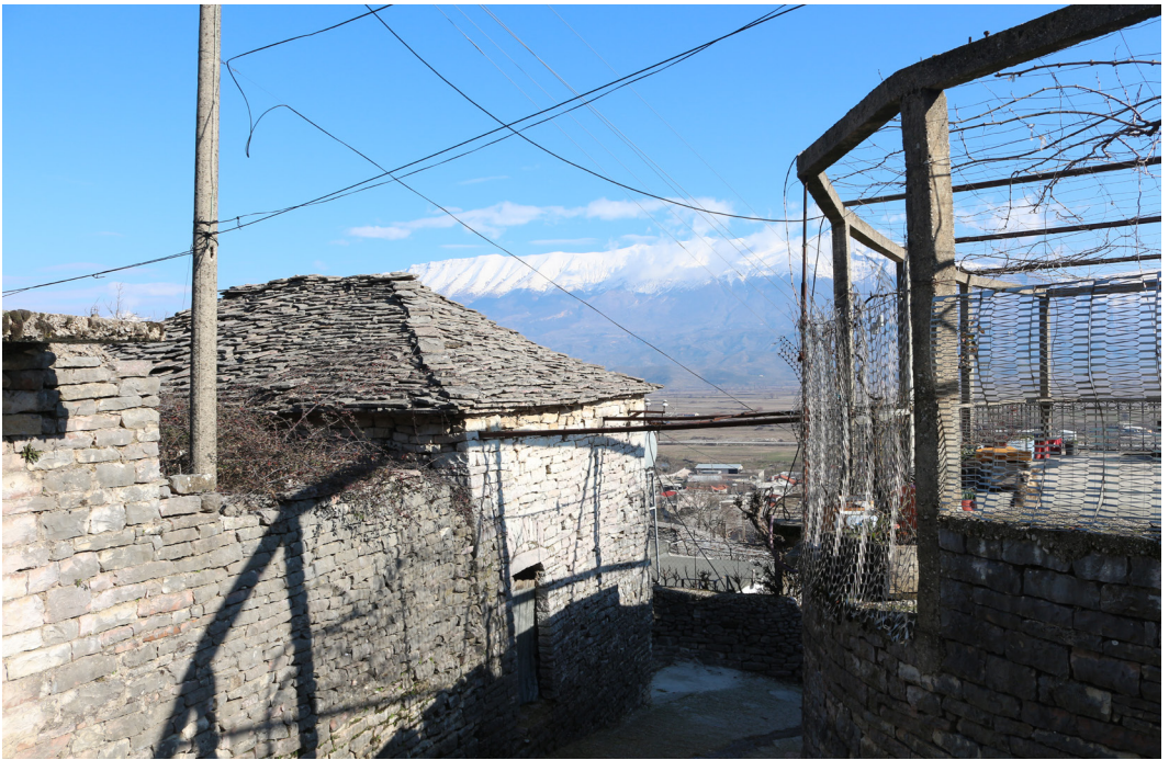
Fig.4 / Example of wrong intervention in the cultural heritage of Deriçan: concrete elements replace ancient structure ignoring one of the restoration principles, the material compatibility. Source / the author.
