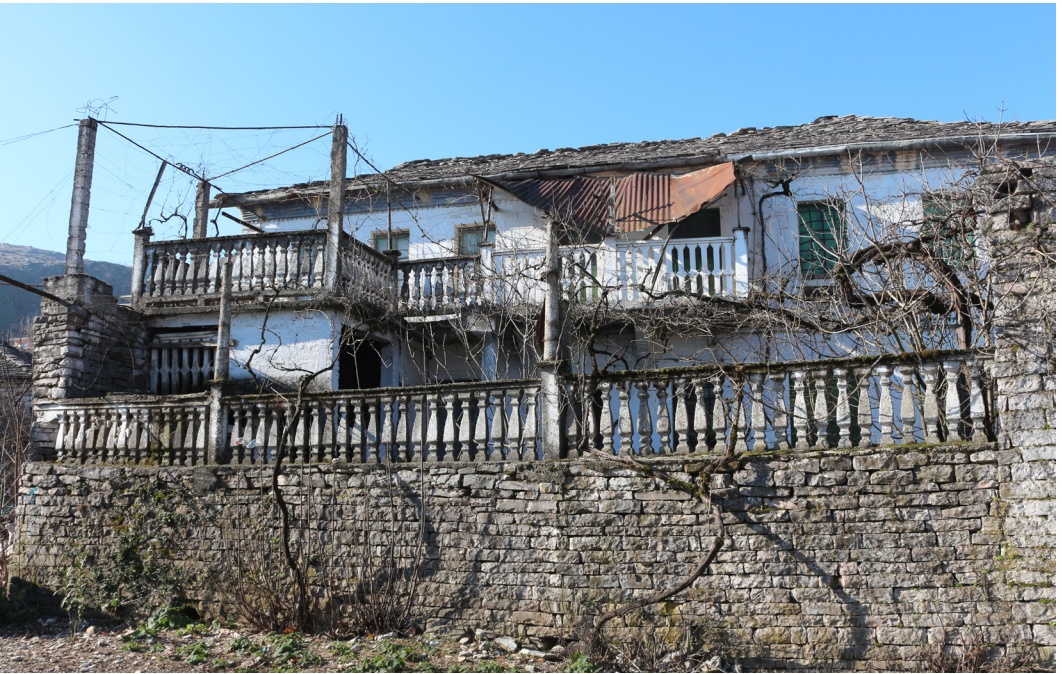
Fig. 2 / An example of historical abandoned buildings in Dervişan. Source / the author.
