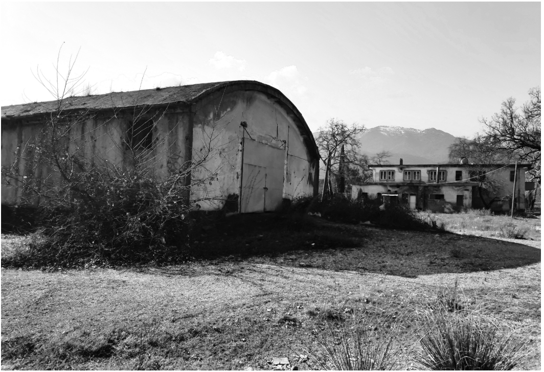
Fig.5 / Abandoned structure. Source / the author
