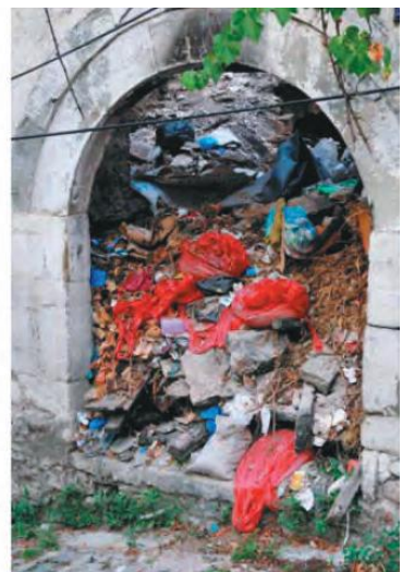
Ruin filled with garbage
