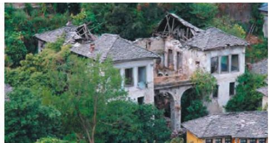
Decayed Gjirokastrian residential building
