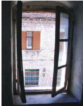
Poor wood quality makes the windows bend
