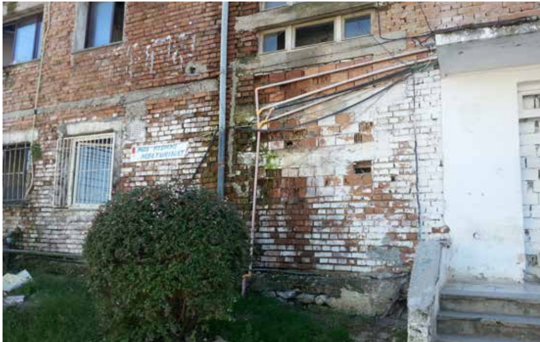
Figure 1 - Wall degradation caused by material deterioration Source - Merita Guri
