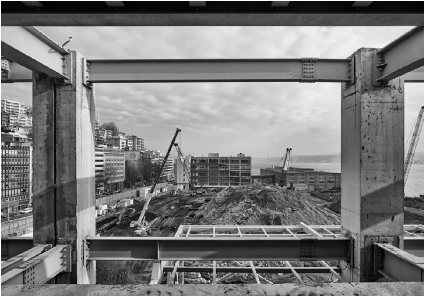
Fig. 6 The Istanbul Painting and Sculpture Museum (Warehouse no. 5) under construction. Photo Cemal Emden
