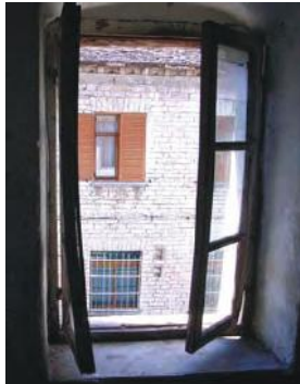
Poor wood quality makes the windows bend
