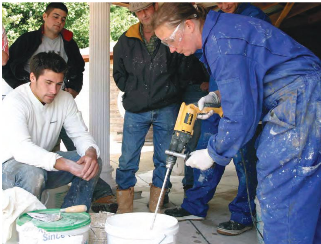
Scottish craftsmen mixing mortar together in the Scottish Lime Centre. Photographer: Roz Artis Young.
