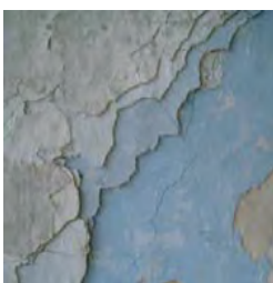
Layers of plaster and paint give clues to which part of the house is the oldest. A light blue color appears on many walls.
