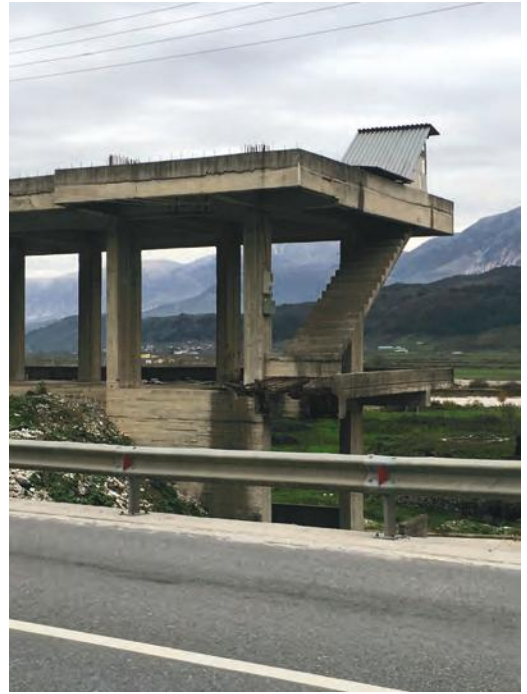
Fig. 4 / Unfinished building in the industrial area of Gjirokastra, typology C. Source / the author
