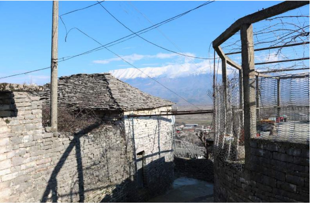
Fig.4 / Example of wrong intervention in the cultural heritage of Deriçan: concrete elements replace ancient structure ignoring one of the restoration principles, the material compatibility. Source / the author.
