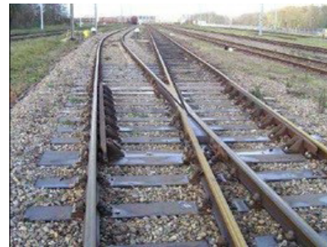
Figura 1. Linjë me traversa plastike [ https://www.lankhorstrail.com/en/railroad-ties ]
