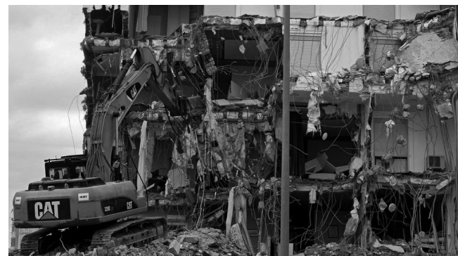
Figure 3. Building Construction after Earthquake/ source.bbc
