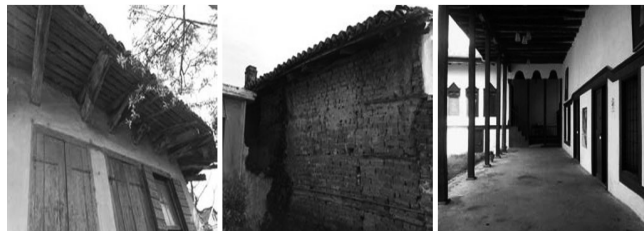
Figure 7 a,b,c. Protruding roof/Wood beams in the external walls/Porch space in front of the house
